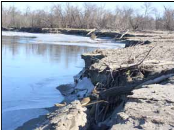
New channel carved by the river. Vegetation alone will not be able to stabilize such a cutbank.
